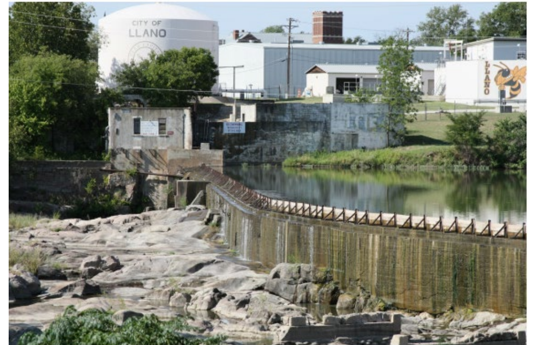
Llano dam on the Llano river sits on the banks of the county seat.
